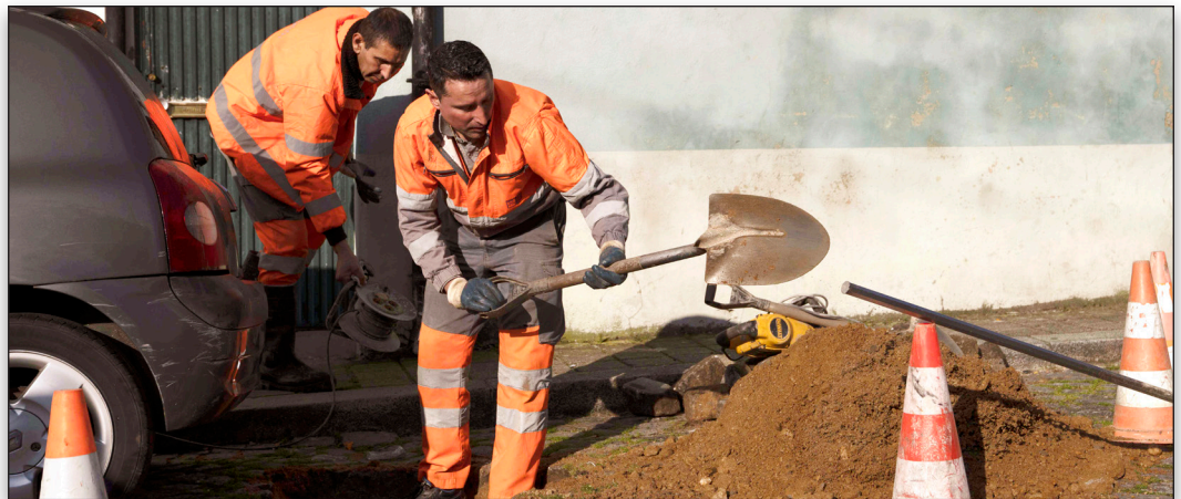
Maintenance quickly respond to issues and update system information while in the field.
